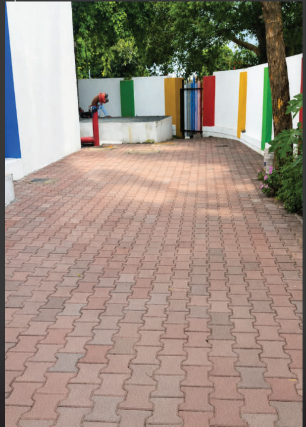
Installation around commercial space in Gandhinagar, Gujarat
